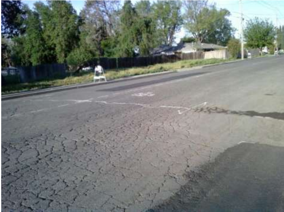
Figure 3. Pre-Construction pavement condition with some skin patching
