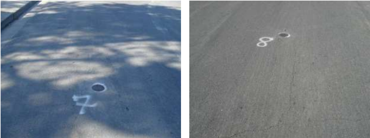
Figure 15. Pavement condition around cores in section 4
