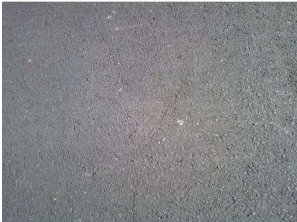
Figure 7. Micro cracks started to show up in product B after 1-2 months of placement
