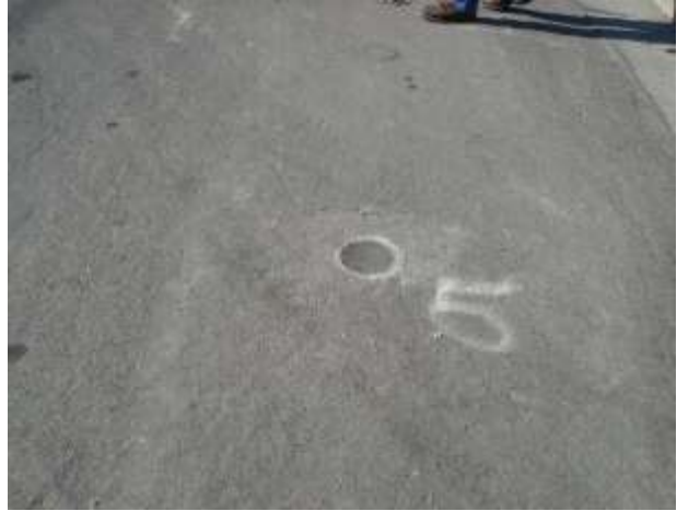
b. pavement condition around core #5
