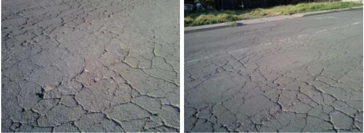
Figure 5. Pre-Construction - Closer look at cracks within the test strip area
