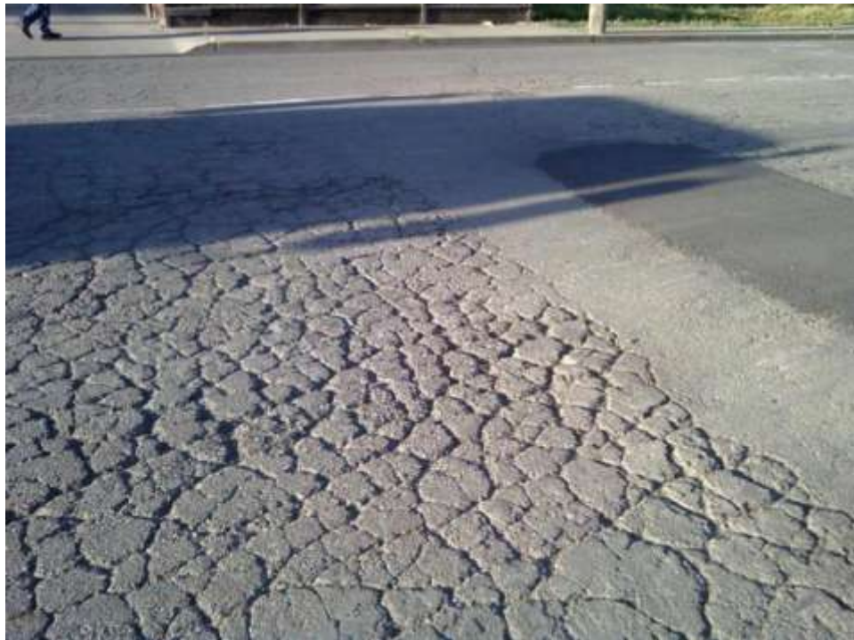
Figure 2. Pre-Construction pavement had severe level of alligator cracking
