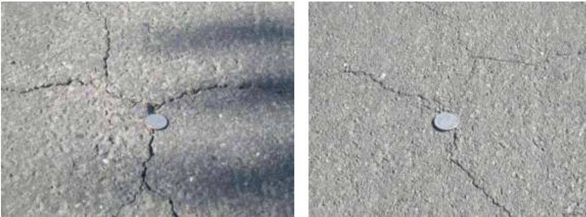
a. Untreated pavement cracks
