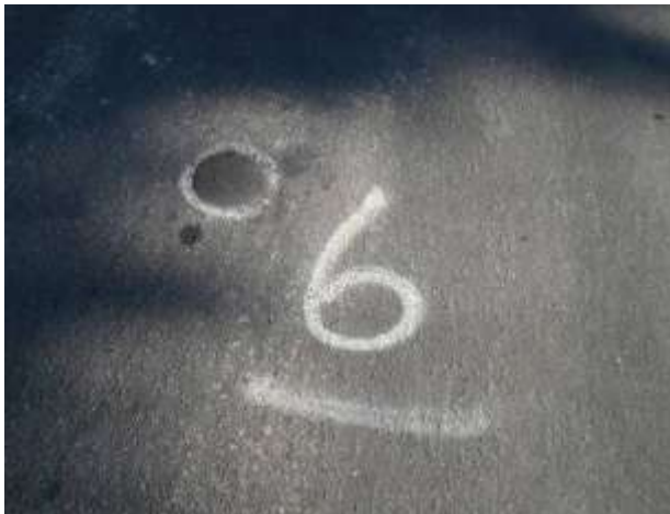
c. pavement condition around core #6
