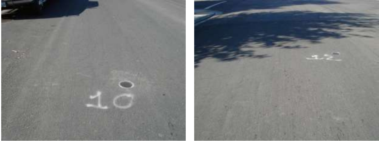
Figure 10. Pavement conditions around cores in Section 2
