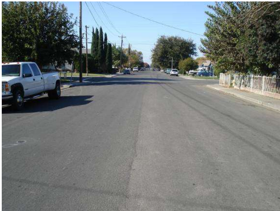
Figure 11. The left of the picture is the Styraflex over fabric
