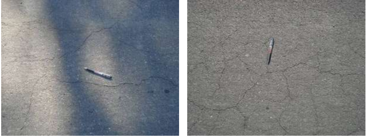
Figure 16. Reflection cracks in section 4
