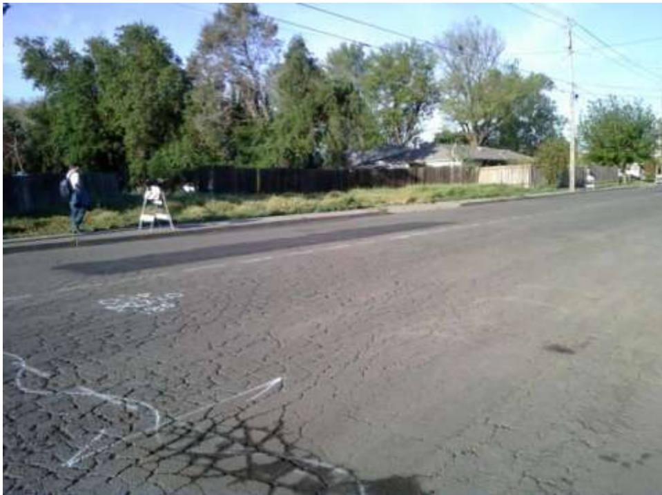
Figure 4. Pre-Construction alligator cracking with patching - Cracks were wide and active
