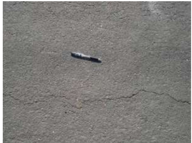
d. Cracks in section 1
