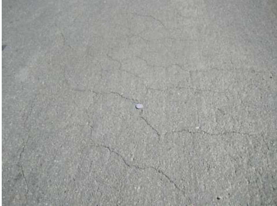
Figure 12. Cracks in the Styraflex with fabric section
