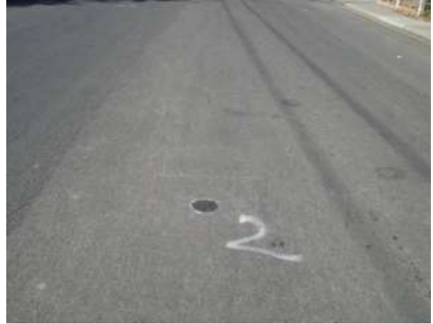
b. Pavement condition around core #2
