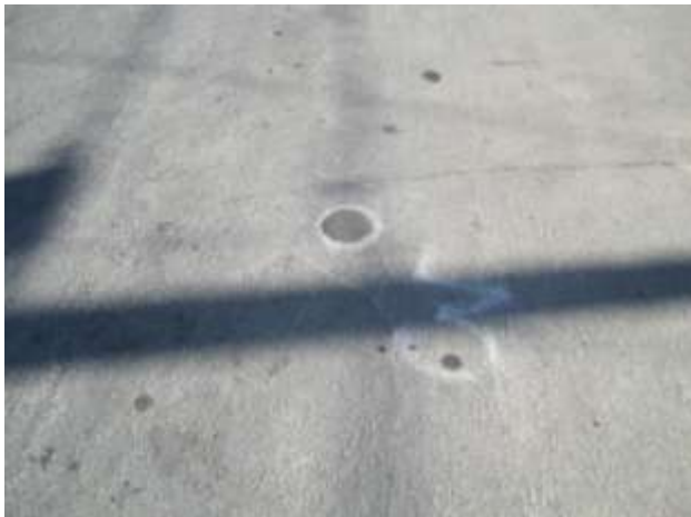
c. Pavement condition around core #3
